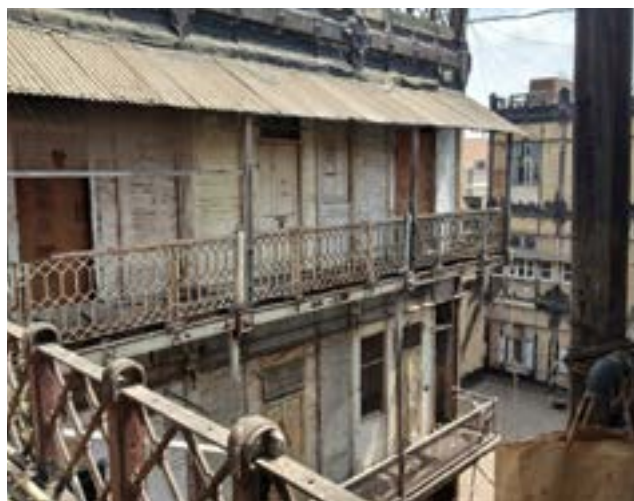
Esplanade Mansion: Top: View from the road shows the frame structure; Centre and bottom: Internal Courtyard, balconies with cast iron railings and other details
